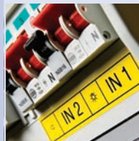
Distribution boxes & patch panels
